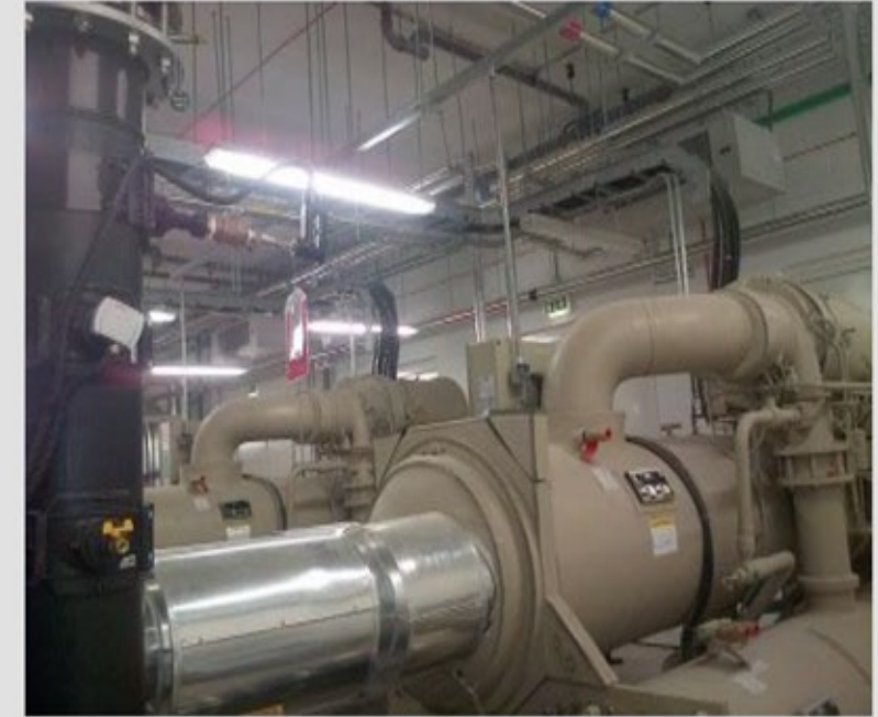
American University @ sharjah ELECTRICAL WORK FOR CHILLER FROM career
