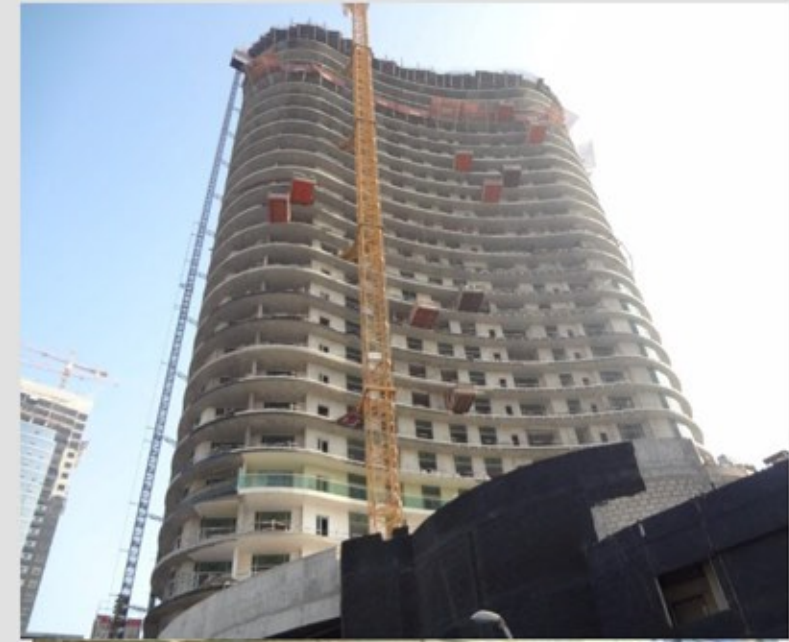
Project Name: Beach Tower Location : Al-Reem Island, Abu Dhabi Description : G-I Duct installation with Thermal Insulation & accessories
